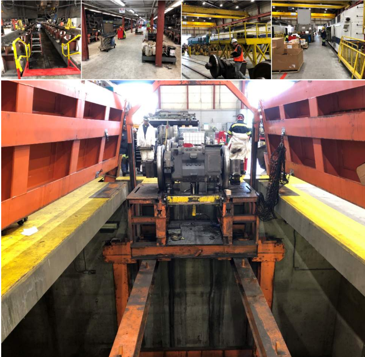
FIGURE 16-2. FIXED FOUR LEVEL WORK AREA ALLOWS COMPLETE LOCOMOTIVE SERVICE IN A SINGLE POSITION
